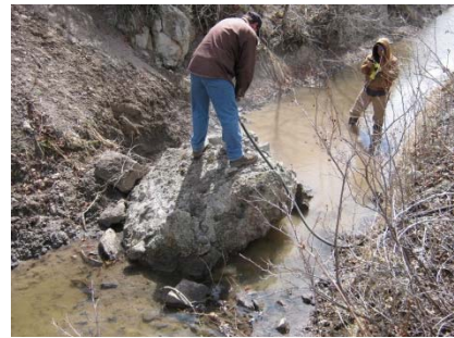
Over 300-ft of air hose and a hammer drill were required to remove this obstruction because there was no access to the canal.
