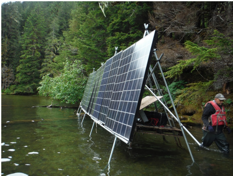
Figure 2. It only takes a dozen 140 watt solar panels to power the remotely monitored video weir at the outlet of Neva Lake, June 14, 2017
