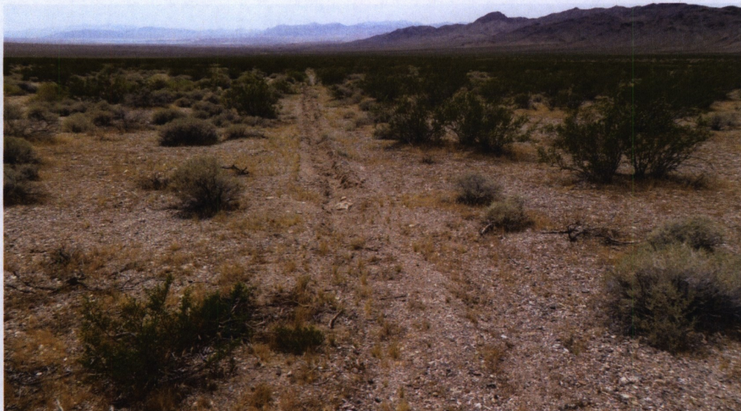
Image 14: Trench and pipe #3 continue southwest toward Fisherman Cove area. Photo looking southwest. Photographed May 10, 2015.
