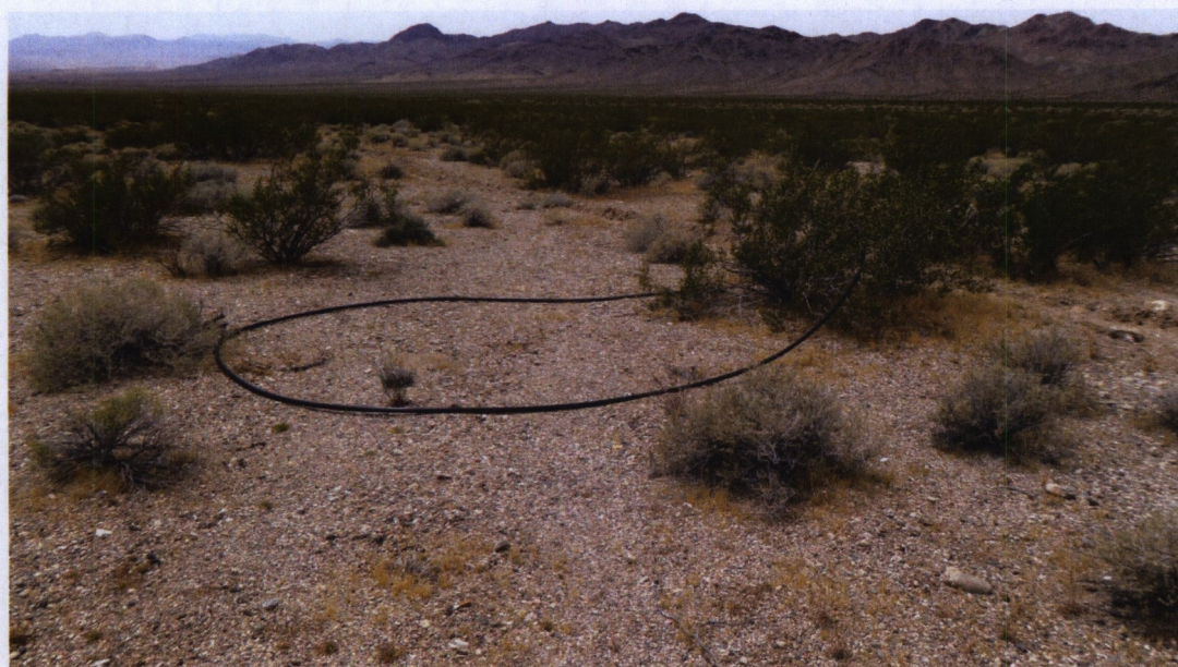
Image 15: Must have been an existing pipe along here and was removed at some point. Followed the trench intrusion to this location 11 S 0749288 4052896. Photo looking southwest. Photographed May 10, 2015.
