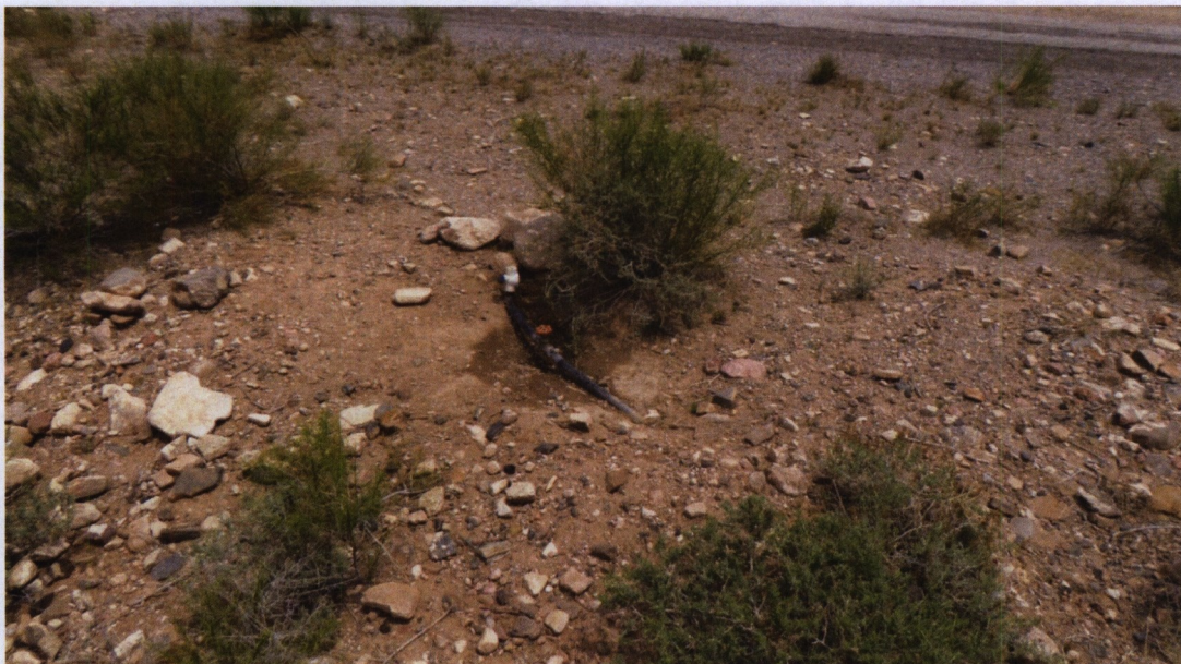
Image 13: Pipe #3 and valves just west of Gold Butte road. Must have used an existing pipe to cross under the road. This pipe and valve have water but the new water trough is still dry. Photo looking east. UTM 11 S 749561 4053233. Photographed May 10, 2015.
