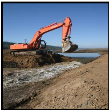
Excavator removes final portion of levee, allowing creekwaters to flow into the Giacomini Ranch's East Pasture.
