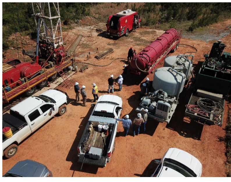
Figure 15: Aerial photo of a crew working on plugging an orphaned well in Louisiana with BIL funds (photo by the contractor, Dynamic) – April 2023 in Union Parish, Louisiana.
