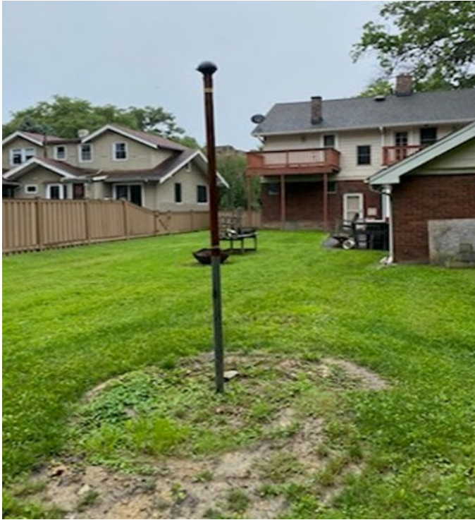
Photo Description: Picture shows a vent installed in a residential backyard prior to plugging. Photo taken during an OWPO site visit.
