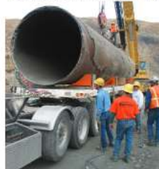
A portion of AA-1 pipeline had to be removed after the 2000 landslide.
