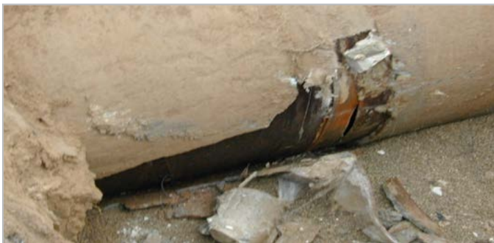
Photo of a Break in the AA-1 Pipeline
