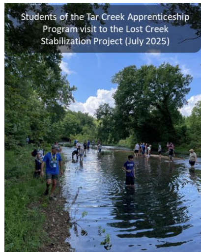
The Lost Creek Streambank Stabilization Project is intended to stabilize the streambank, reduce land loss, and provide safe access for recreational opportunities. Tar Creek NRDA, Oklahoma. Photo Credit: DOI
