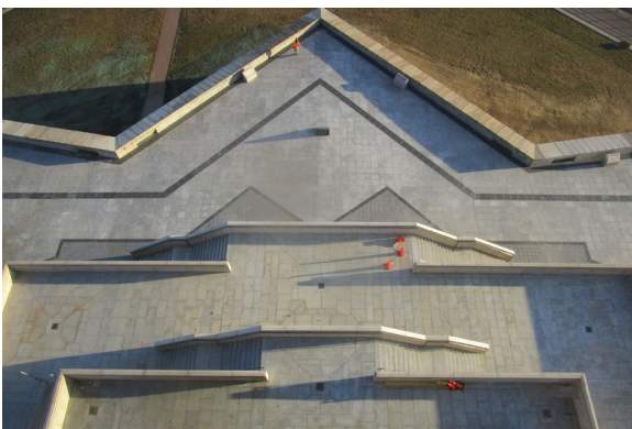
An aerial view of the completed terreplein repairs at Fort Wood at the base of the Statue of Liberty. Photo Credit: NPS
