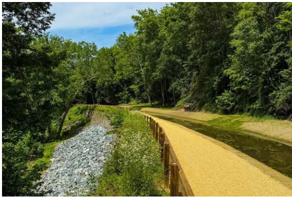
The log wall after stabilization at Chesapeake & Ohio Canal National Historical Park. Photo Credit: NPS
