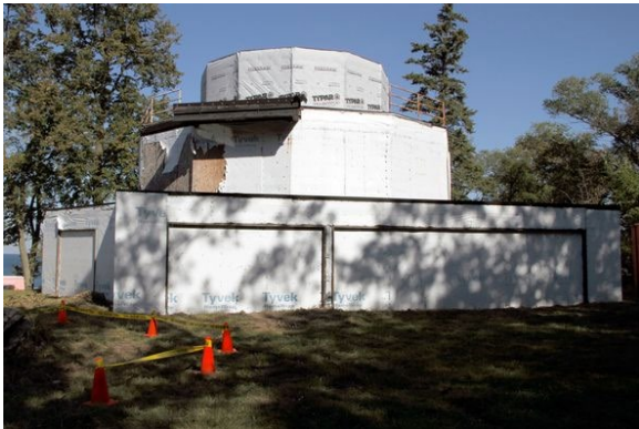
Renovations to the House of Tomorrow in progress. Photo Credit: Katrina George
