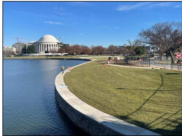
Figure 2 – Completed repairs to the seawall at Tidal Basin reservoir. Photo Credit: NPS
