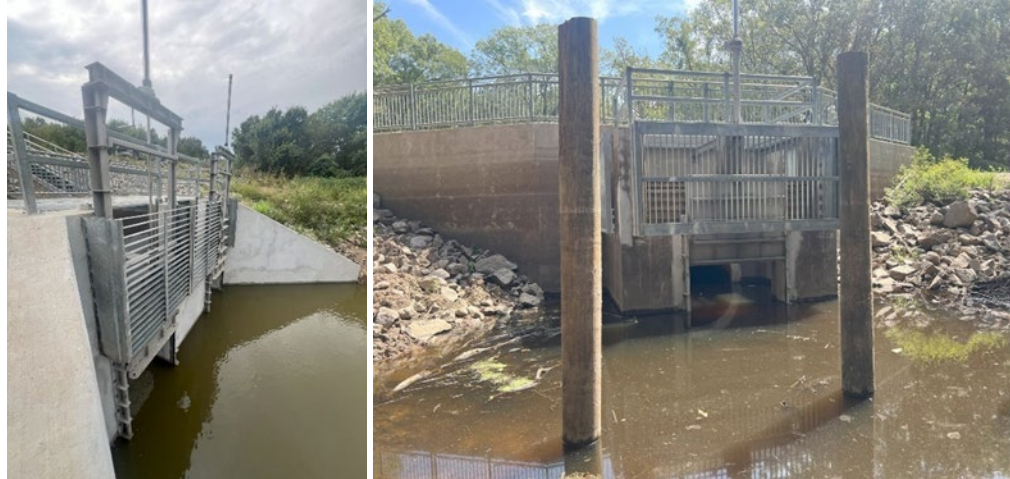
Dale Bumpers White River NWR: Replaced Water Control Structures to Control Flooding for Improved Visitor Access and Hunting Opportunities. Image: USFWS
