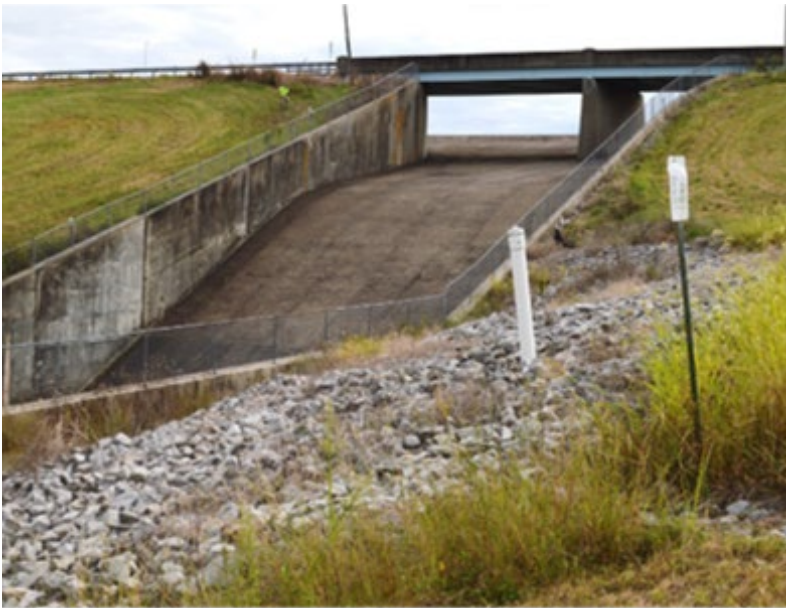
Little Grassy Dam Service Spillway, Crab Orchard, NWR, IL. Planning for rehabilitation is currently underway with a cooperative agreement between Region 3, NWRS and the USACE. Credit: USFWS
