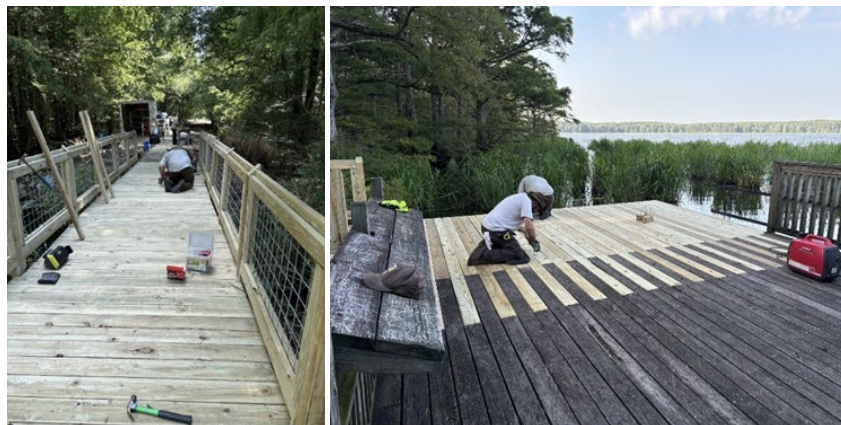
GAOA Funded Maintenance Professionals Repairing a Damaged Fishing Pier at Wappanocca NWR. Image: USFWS
