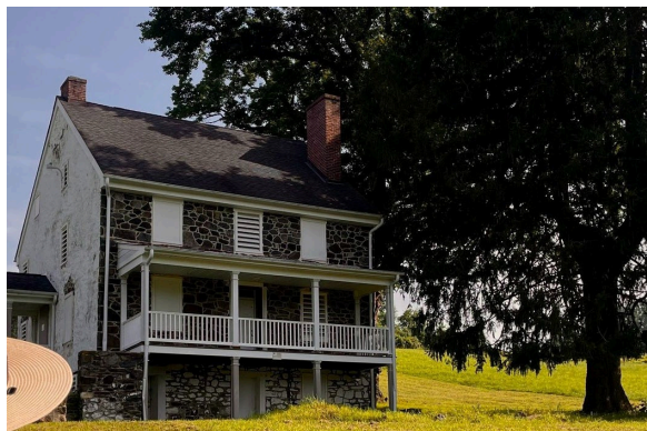
Ramsey House at First State National Historical Park before GAOA LRF repairs. Photo Credit: NPS
