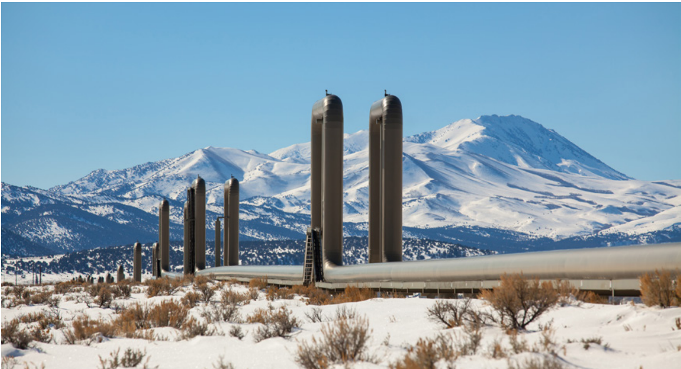
Geothermal pipelines in Nevada.
