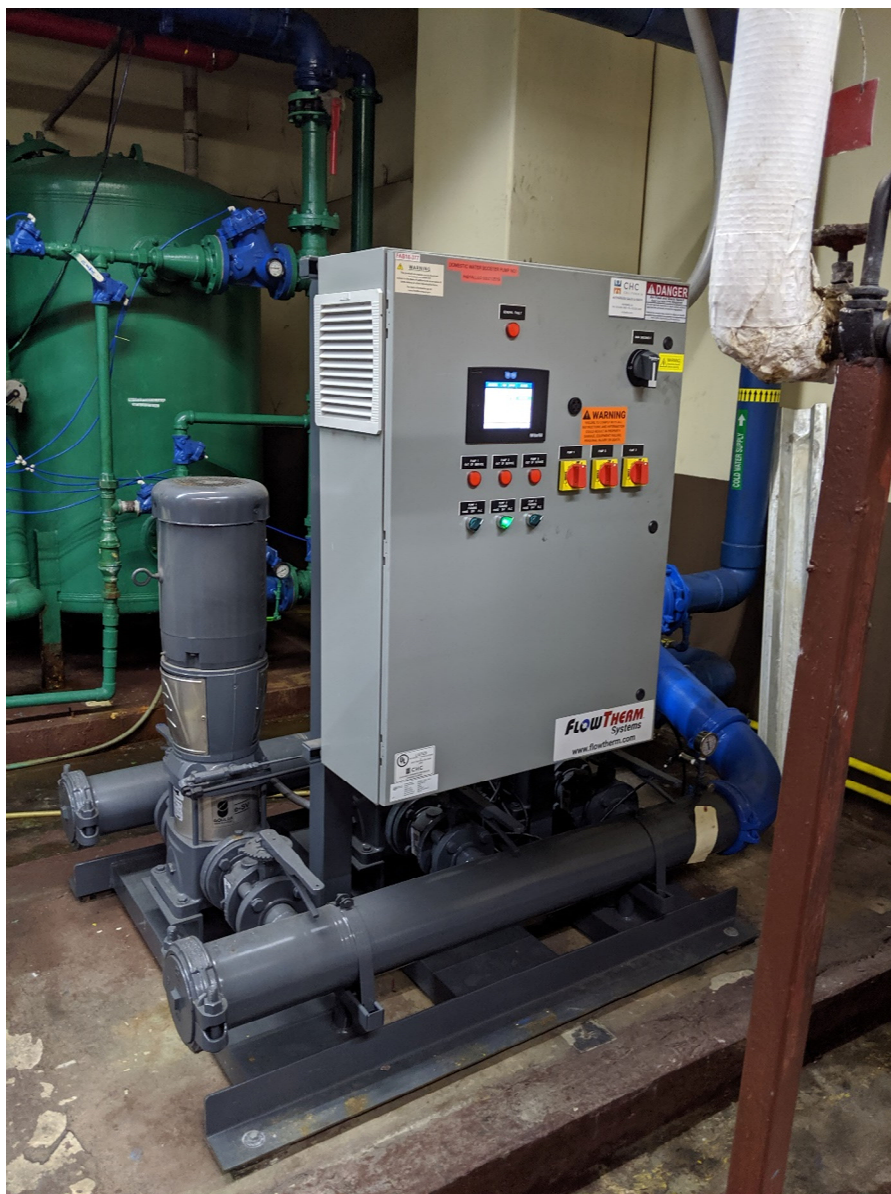
Domestic water pumping unit
