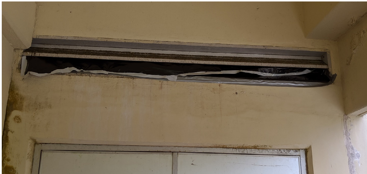
Blocked off outside air intake
