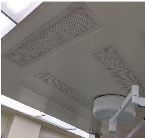
OR ceiling showing inadequate coverage
