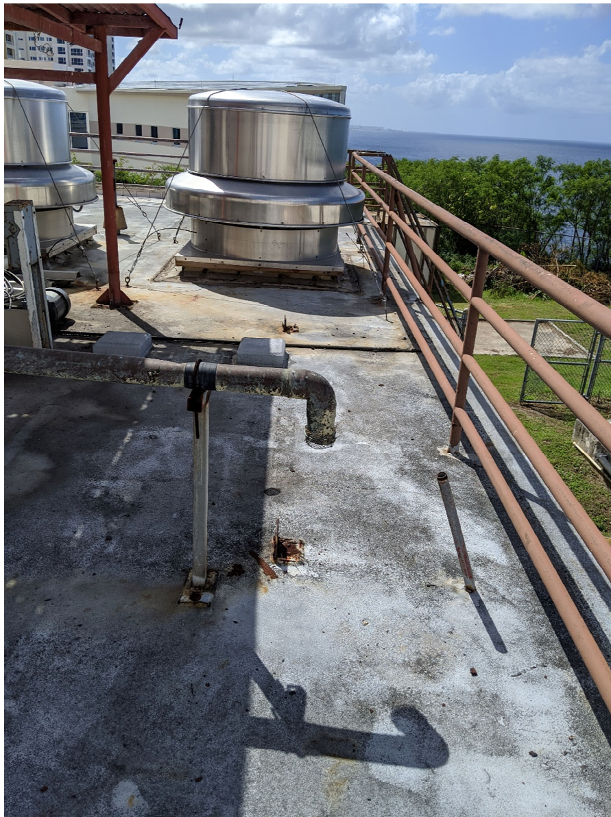
Medical air inlet closer than 25 ft. from exhaust fan discharge
