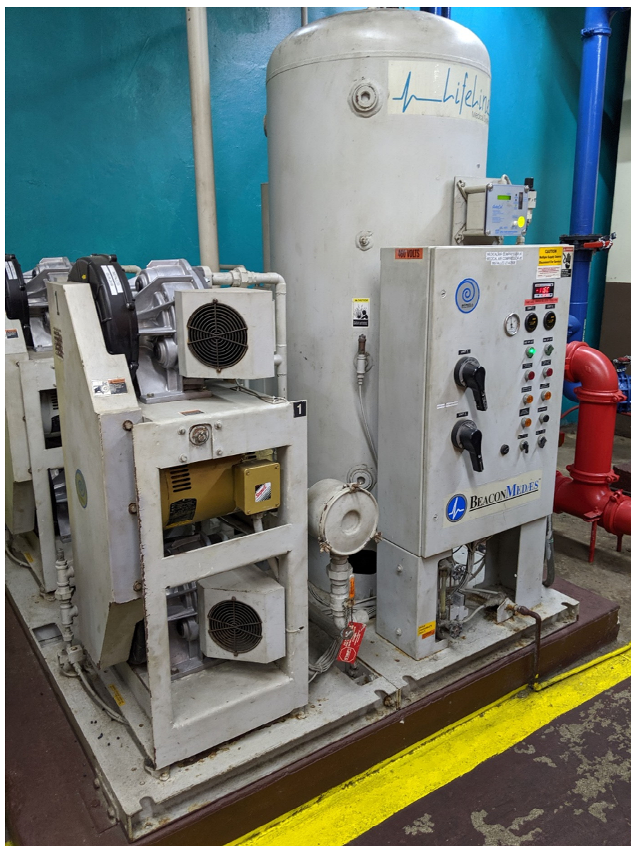
Medical air compressors with 20,000 gal water tank beyond
