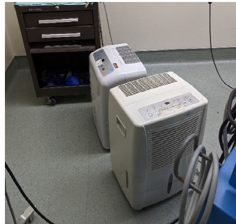
Portable dehumidifiers being used in ORs
