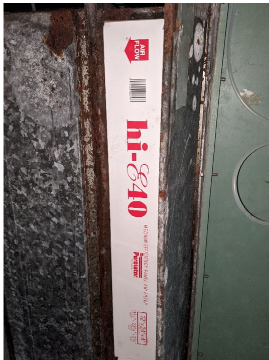
MERV 8 filter, typical of all air handling units observed.
