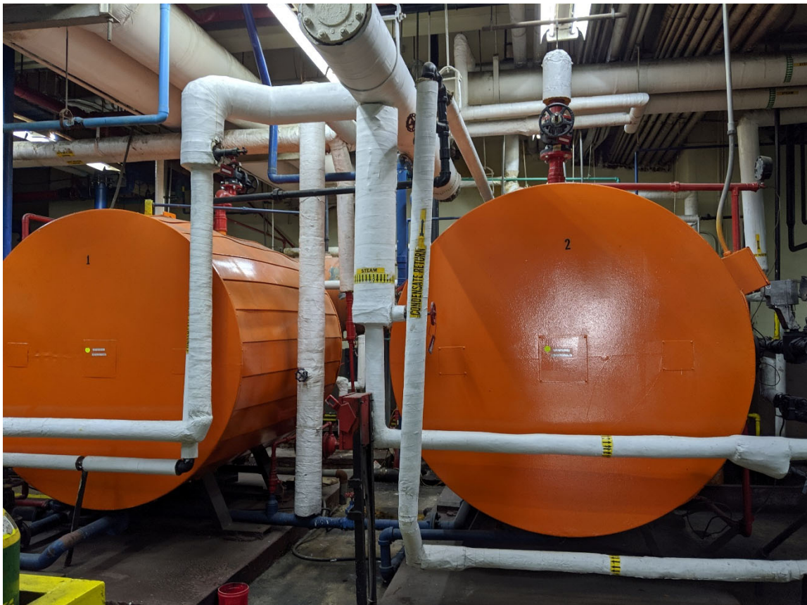
Domestic hot water heat exchangers
