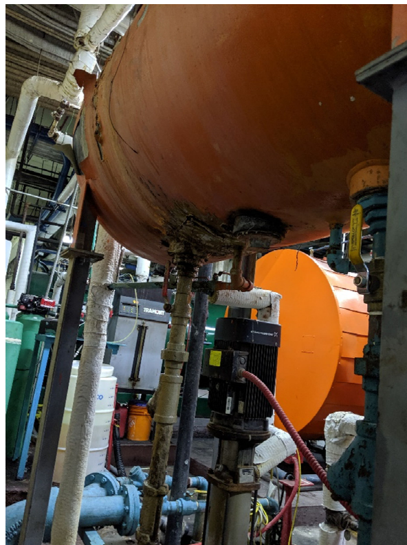
Boiler feedwater/condensate receiver tank
