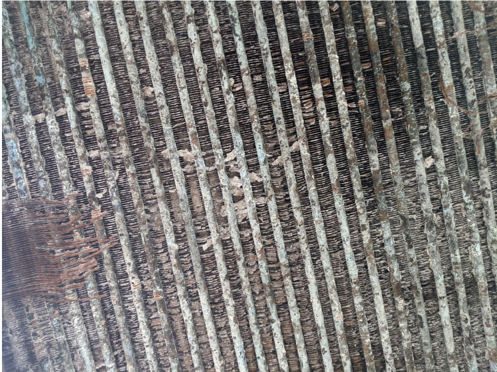
Corroded emergency chiller condenser coils
