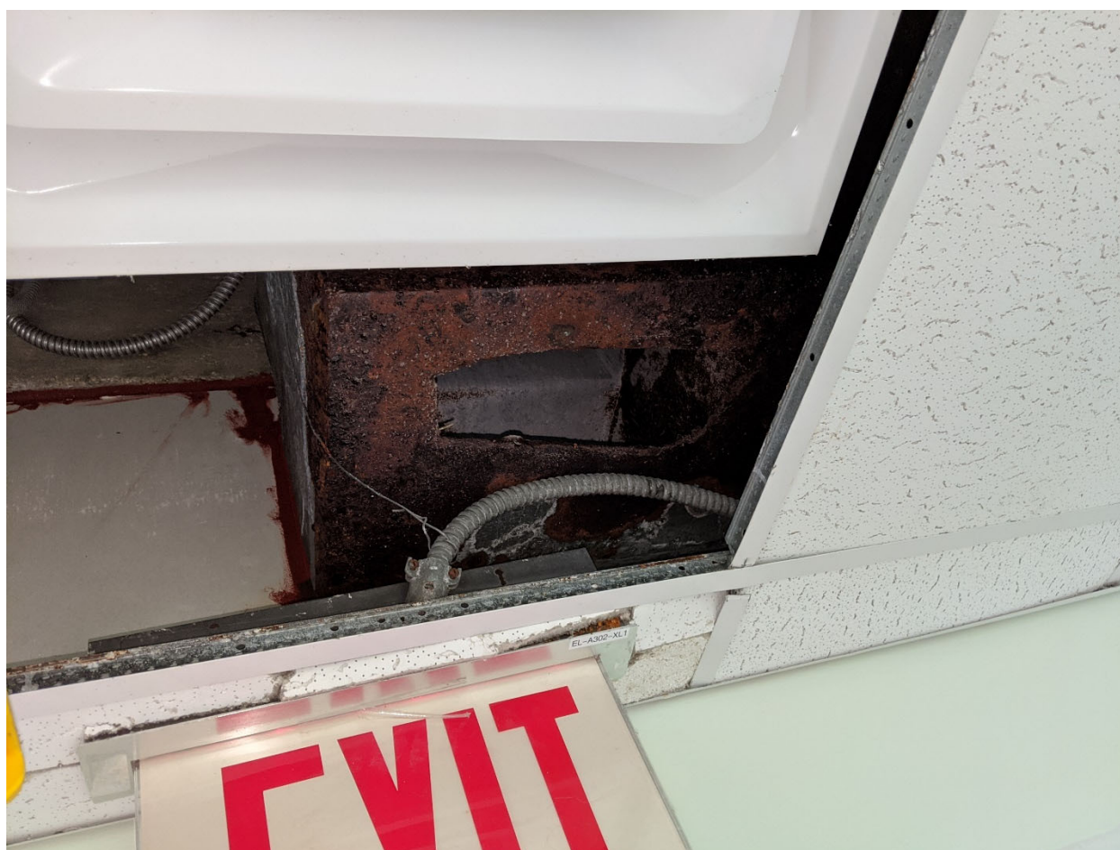
Corroded outside air ductwork drawing air from inside the building.
