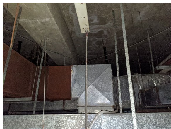
Inappropriate kitchen exhaust duct material
