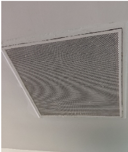
Access panel/grille into patient bedroom soffit space
