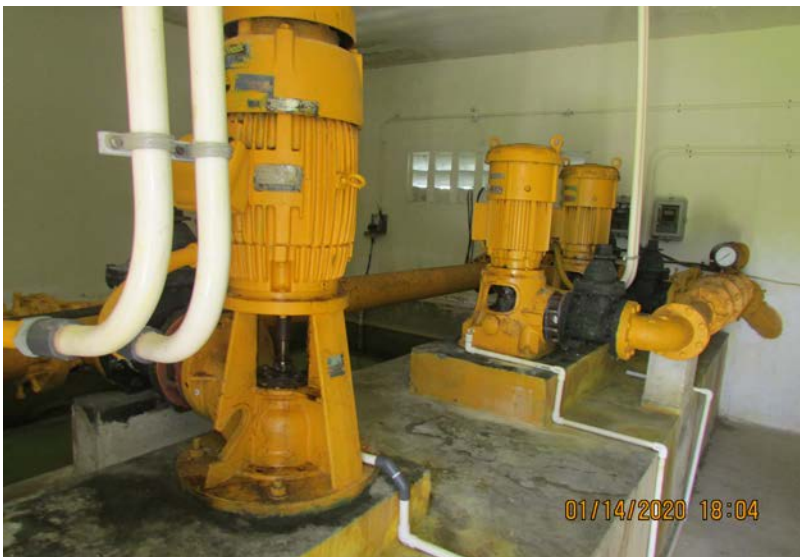
Figure 5: Laura Pump Station with three pumps (Reclamation photo 2020).
