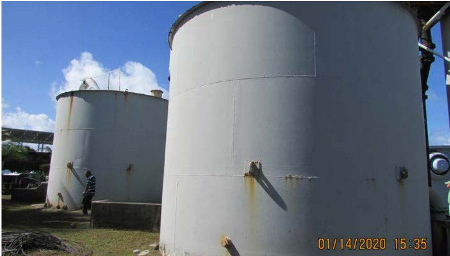
Figure 7: Two automatic valveless gravity filters at WTP C (Reclamation, 2020).
