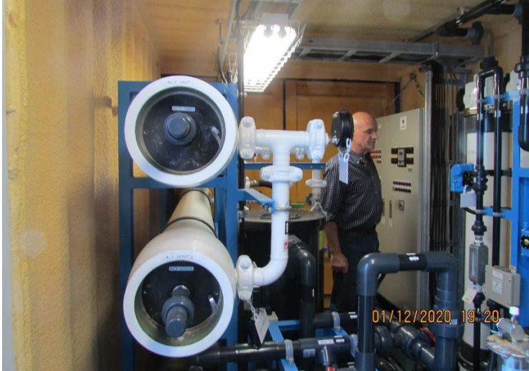
Figure 11: RO units for hospital water (Reclamation, 2020).
