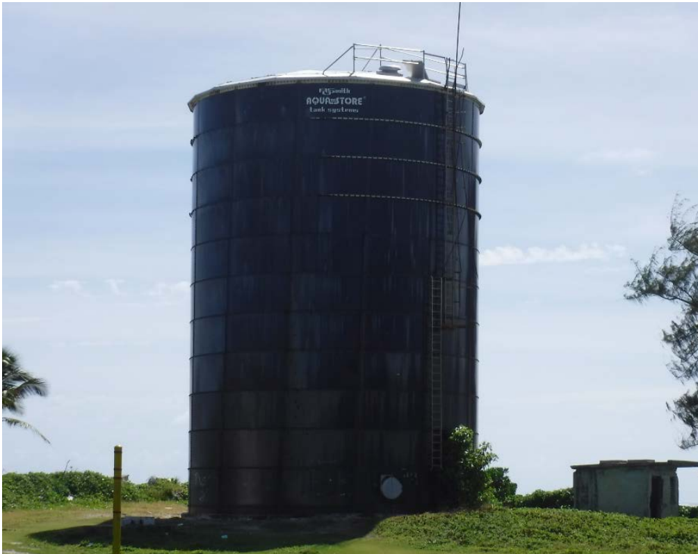
Figure 15: Abandoned 400,000-gallon standpipe (Reclamation, 2020).
