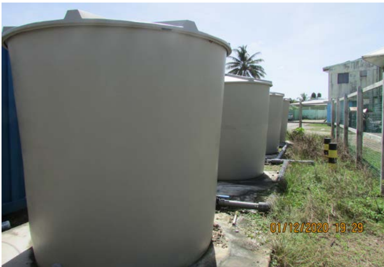
Figure 12: Storage tanks for water treated with RO (Reclamation, 2020).
