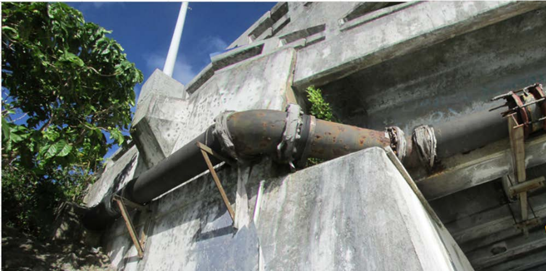
Figure 27: Ductile iron pipe with wrapped joints at bridge crossing.
