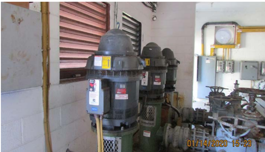
Figure 9: Three pumping units at WTP C. Each pump is rated for 162 feet of head and 800 gpm (Reclamation, 2020).
