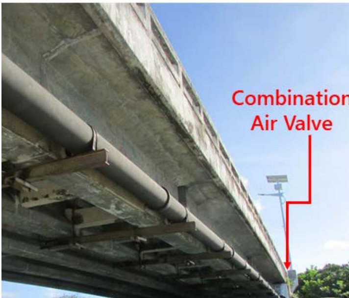
Figure 32: Place an air valve at the bridge abutment, rather than the actual high point.
