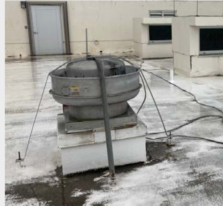
Hurricane straps on rooftop equipment
