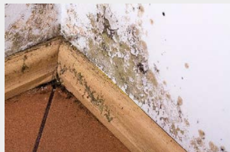
Mold damage due to moisture intrusion
