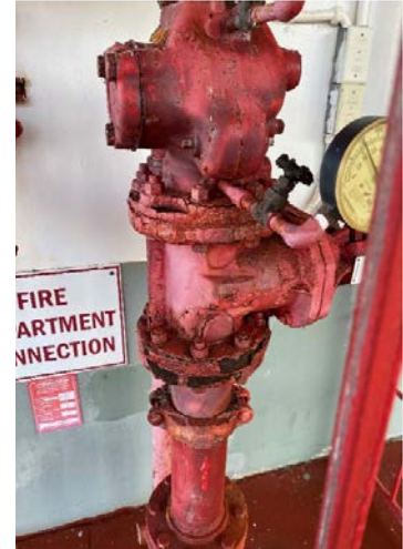
Figure 5-14: Cyclone Corroded fire protection system. Taken from Guam School Assessment, USACE, 2021
