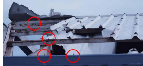
Failure of roof fasteners due to corrosion
