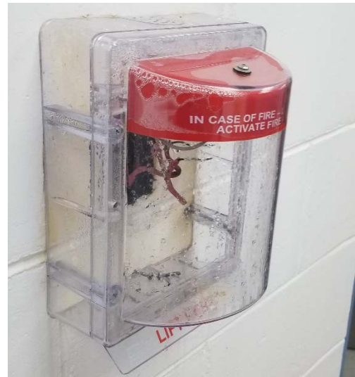
Figure 5-13: Condensation in fire alarm caused by improper sealing of enclosure
