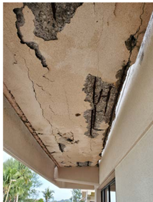
Figure 5-10: Spalling of reinforced concrete due to lack of concrete cover causing corrosion in the steel reinforcement
