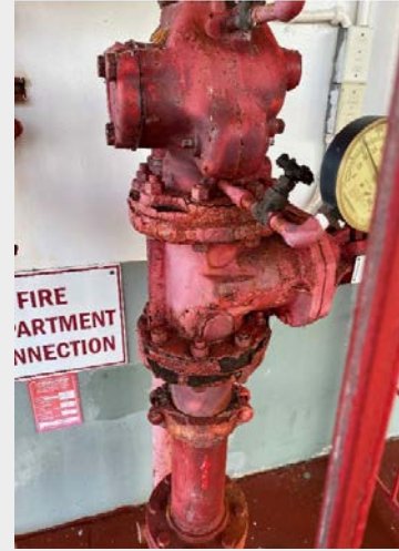
Cyclone corroded fire protection system. Taken from Guam School Assessment, USACE, 2021
