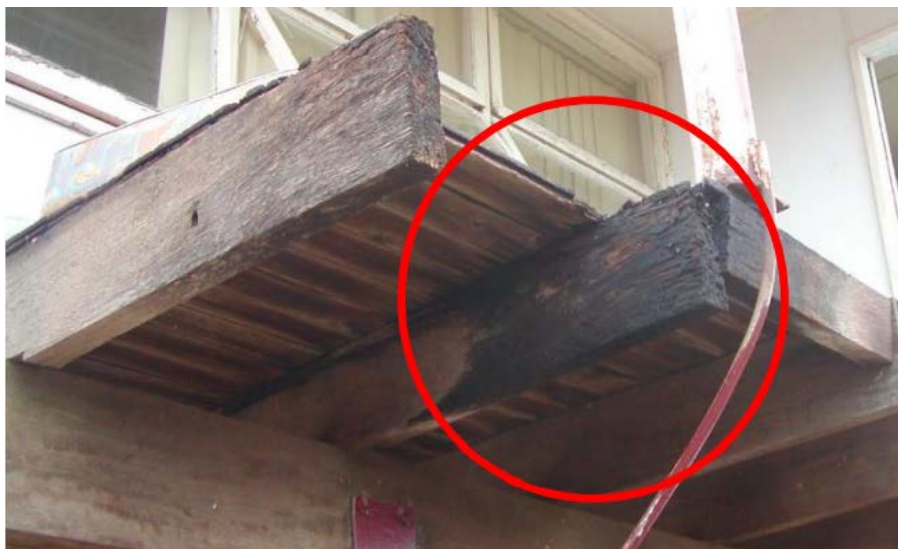
Figure 5-11: Rotting of untreated, unprotected timber (Department of Fire & Emergency Services, 2022)
