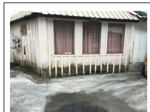
Figure 5-2: Moisture damage without adequate eaves, gutters or site drainage (USACE 2019)
