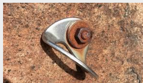
Galvanic corrosion on fastener. Note that the stainless-steel lug is not corroded.
