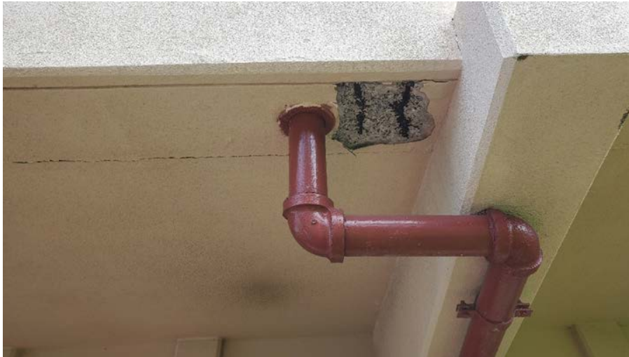
Figure 5-8: Reinforcement corrosion due to lack of cover
