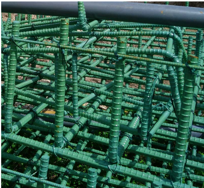
Figure 5-9: Epoxy-coated reinforcing with damage to coating and corrosion
