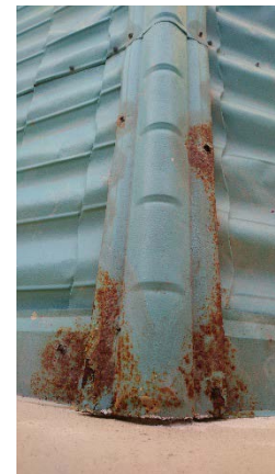
Dissimilar metal corrosion on roof fasteners
