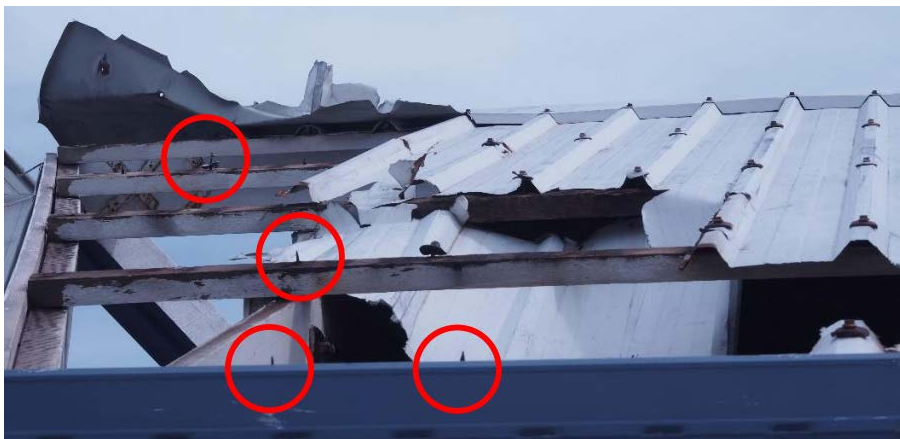
Figure 5-5: Failure of roof fasteners due to corrosion (Department of Fire & Emergency Services, 2022)
