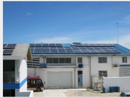
Photovoltaic arrays on building roof
