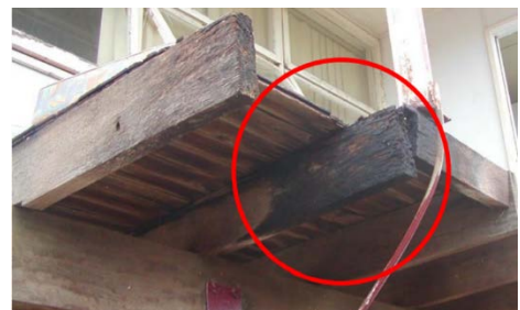
Rotting of untreated, unprotected timber
