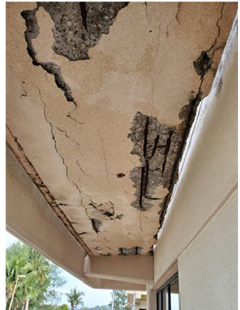
Spalling of reinforced concrete due to lack of cover leading to corrosion of the steel reinforcement
