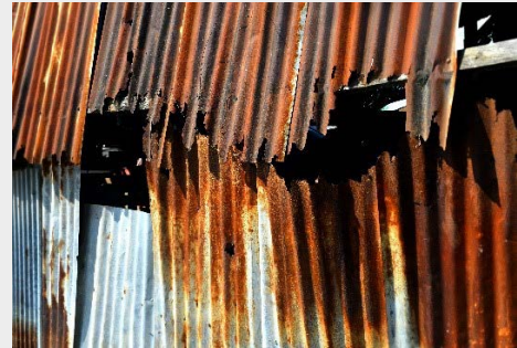
Rusting metal panels due to improper coatings
