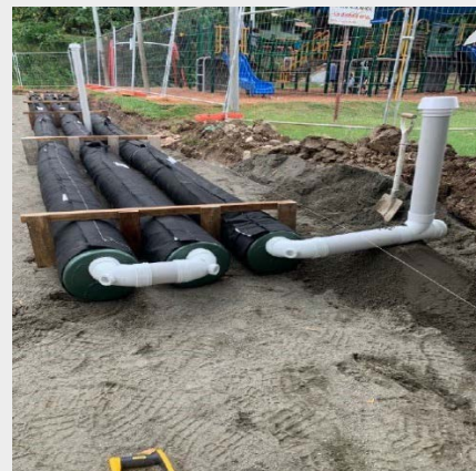
Wastewater Advanced Aeration Bed pipework.
