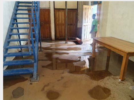
New building flooded from poor site drainage.
