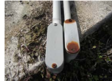
Figure 5-1: Example of corrosion of dissimilar metal fastener
