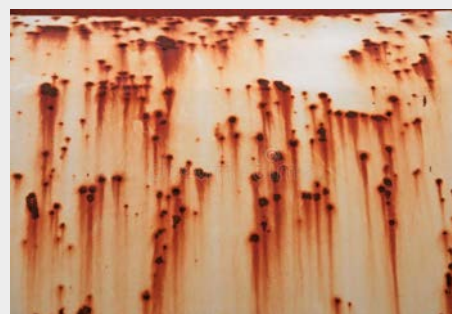
Rust on a painted surface
