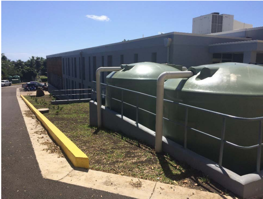
Figure 4-11: Rainwater harvesting tanks on new building in Rarotonga
