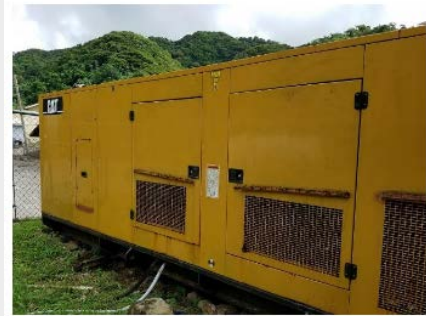
Temporary Diesel Generator Taken from Appendix C, Electrical LBJ TMC,
