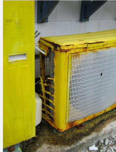
Corrosion on HVAC equipment located at seaward side of the building
