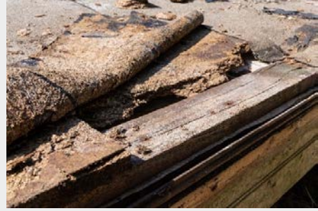
Swollen OSB due to moisture intrusion
