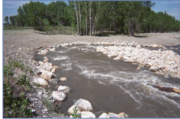
Bio-engineered fishpass enables fish to safely and effectively pass around low-head diversion dams.
