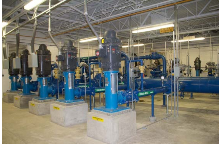
Fort Peck Water System, Fort Peck Montana
