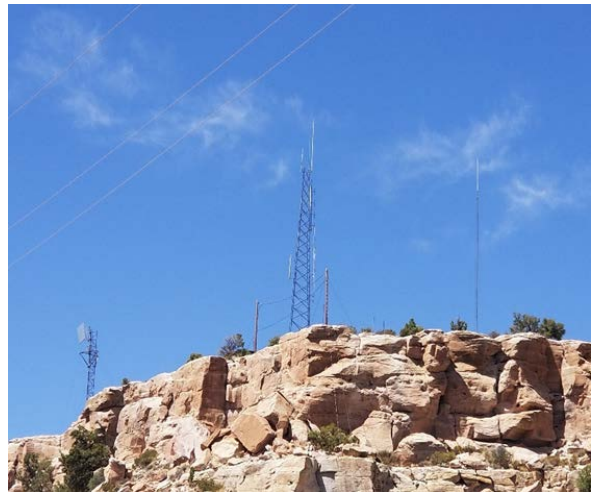
Telecommunications Tower, Keams Canyon Arizona
