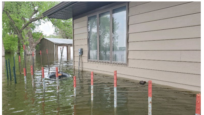
Figure 2. Lake Andes NWR – Examples of Flood Damaged Facilities to be Replaced with GAOA Funding
