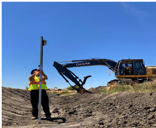
Figure 3: Checking Grades on a Canal Rehabilitation Project at San Luis NWR, California
