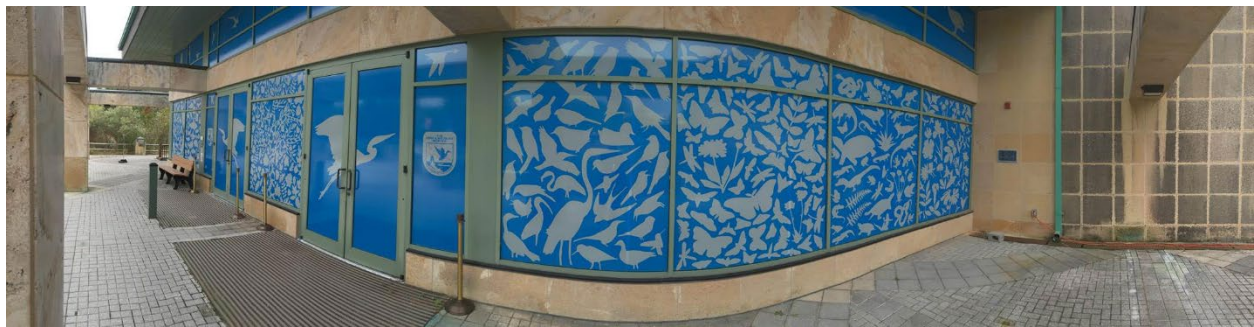
Bird-friendly window treatments, seen here at Patuxent National Wildlife Refuge Visitor Center, can be attractive, low-cost, effective measures to reduce bird-building collisions. Credit: USFWS
