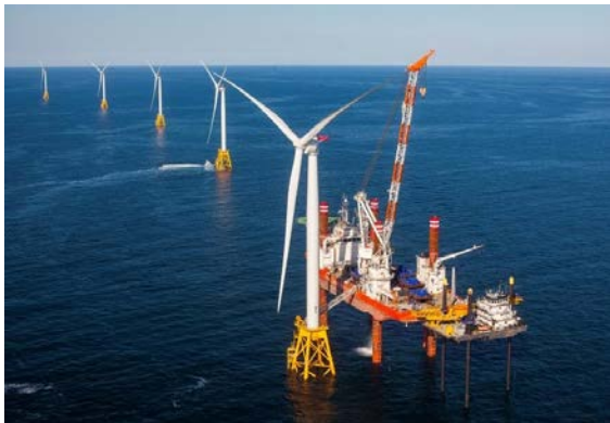
Block Island Wind Farm
