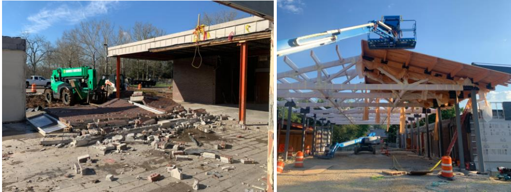
Left: Selective demolition of original lobby. Right: New lobby and roof under construction.
