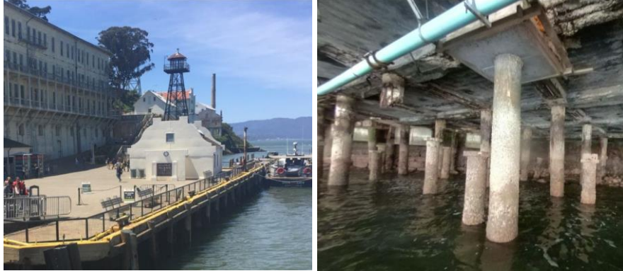
Left: The Alcatraz fixed wharf with visitors waiting for ferry. Right: Deteriorated wharf structure below.
