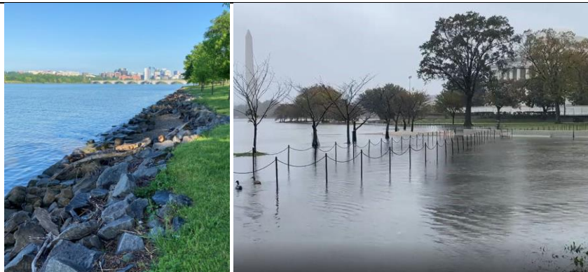
Left: Existing West Potomac Park seawall during low tide. Right: Tidal Basin seawall and public walkways flooded during high tide.
