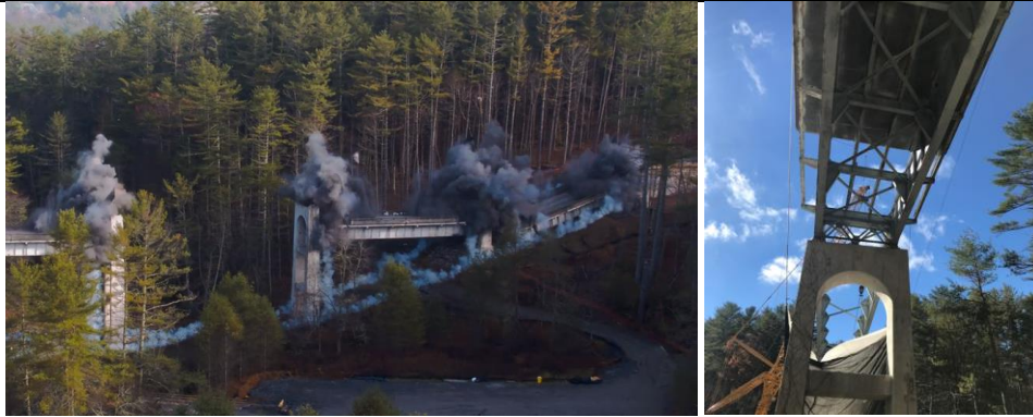
Left: Demolition of the old bridge. Right: Construction of the replacement bridge.
