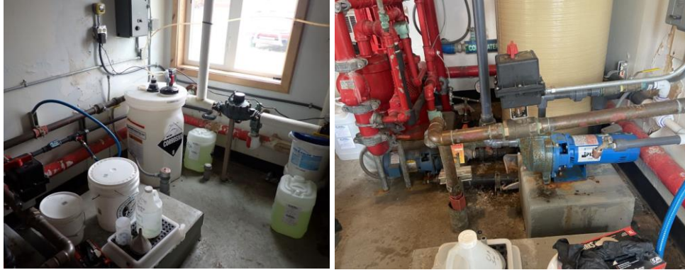
Left: Hazardous chemical storage needed to treat high mineral content raw water.
