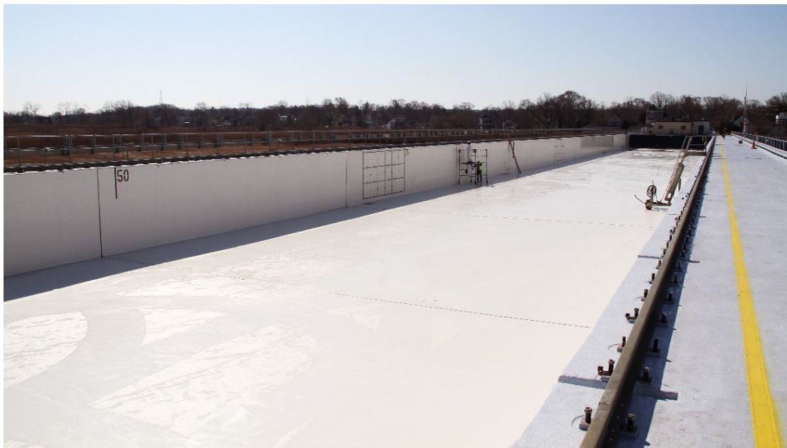
Figure 7. View of empty tank showing fresh paint, concrete repair, and new sealants prior to it being refilled with Sandy Hook Bay seawater in a three-day operation. (Photo from Mike Brenna, BSEE)
